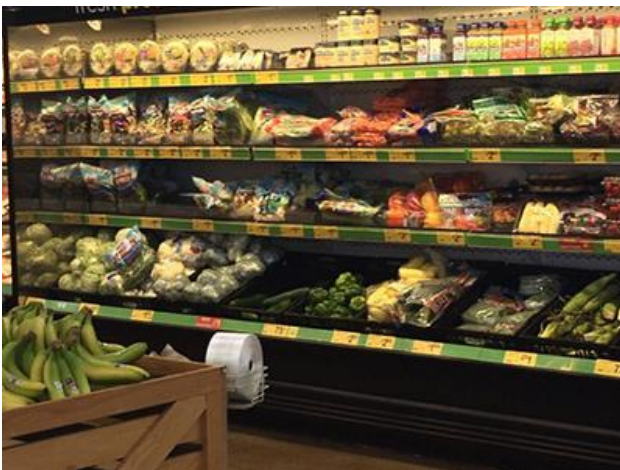
Older, low-capacity coolers
